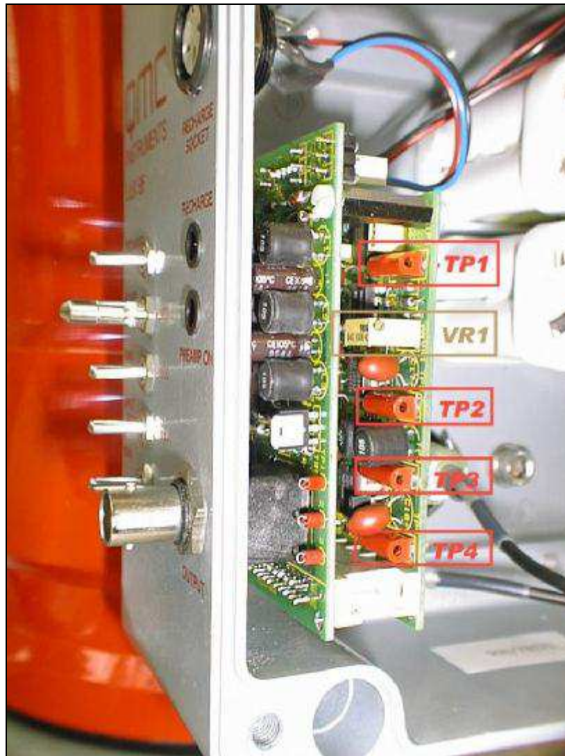
Photo 5.3. View of the switchboard and amplifier circuit board identifying the voltage test points and multi turn potentiometer
